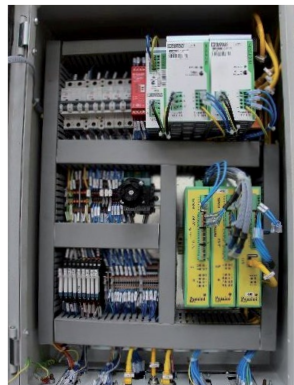
▶ Inspektor Electrical Cabinet
